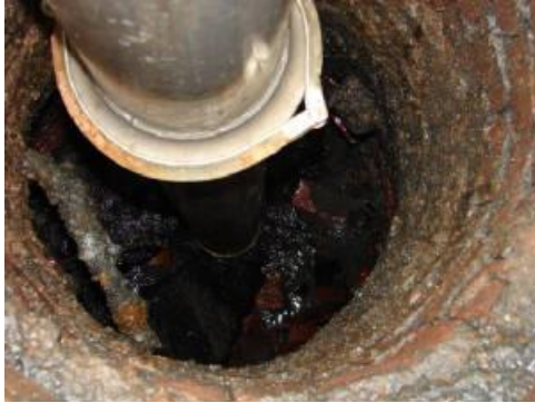
Man Hole Prior to Repair
