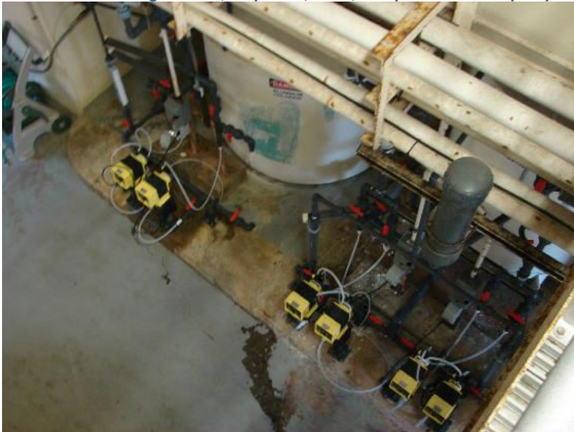
Chemical Feed System Installation
