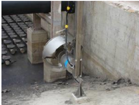
Mixer Prior to Removal for Inspection and Routine Service
