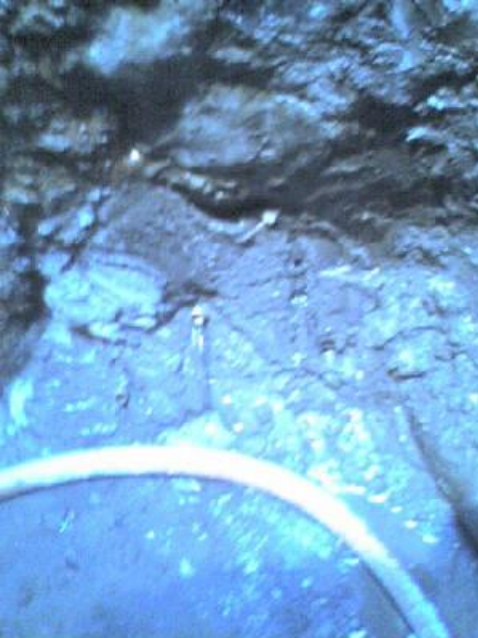
Leaks Through the Walls of a Pump Station Prior to High Pressure Chemical Injection Grouting
