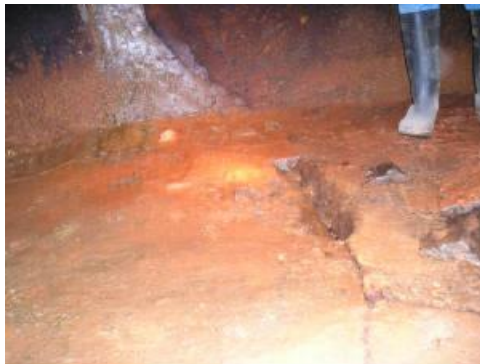
Crack in Tank Floor Prior to Repair - over 100,000 gpd of Water Lost Through Crack
