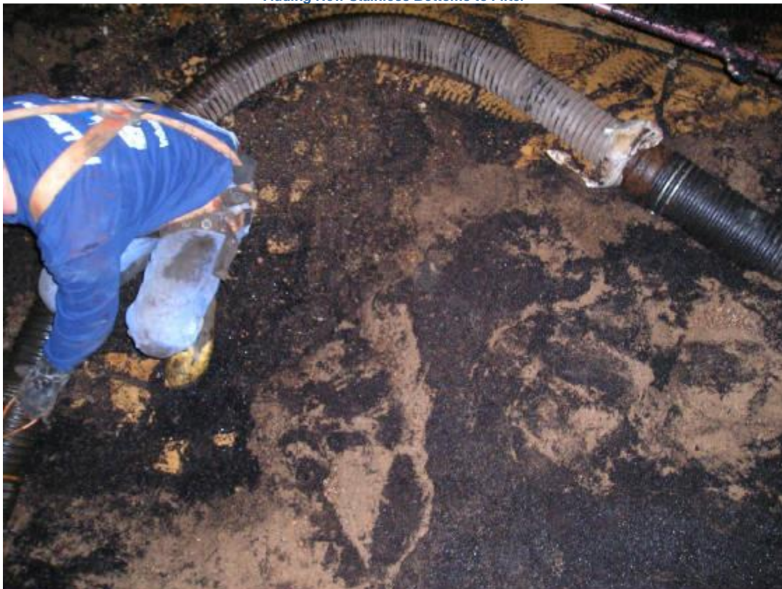
Removing Media From Water Plant Filter Prior to Repairing and New Media Addition
