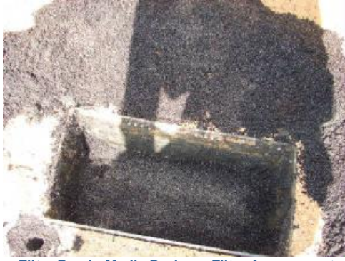
Filter Box in Media During a Filter Assessment
